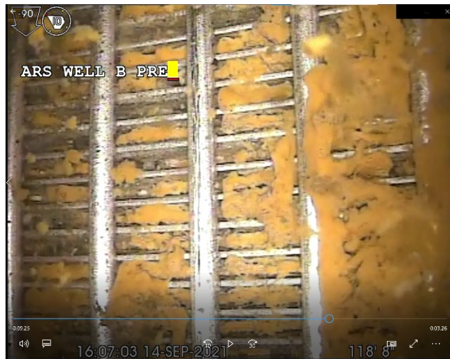
Injection Well B before rehab
